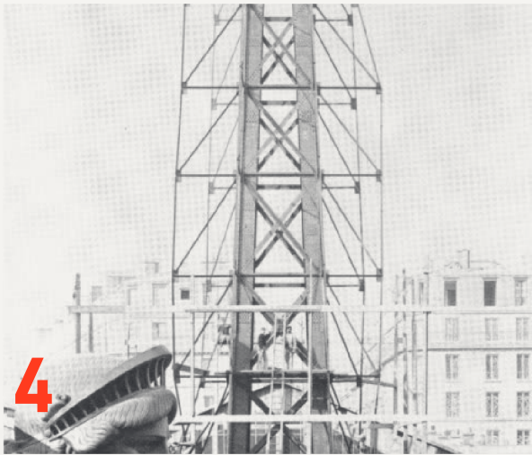
Plate 4 — The statue under assembly. The scaffold outside will go; the skeleton inside will not.
